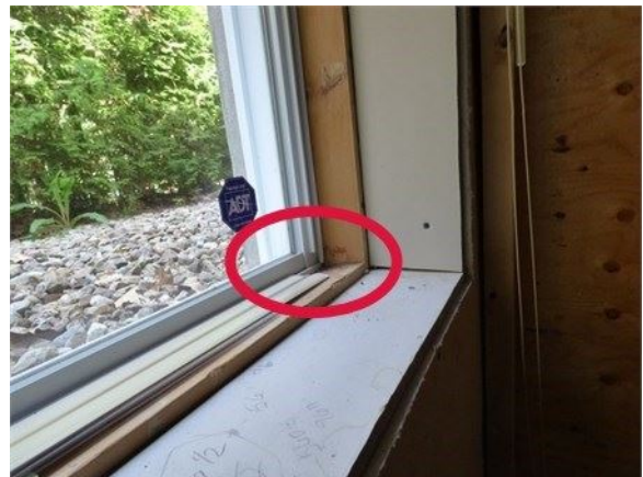
Water leak noted
