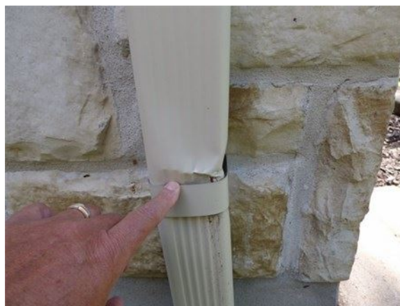
Replace damaged downspout
