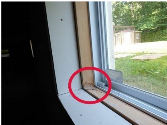
Water leak noted
