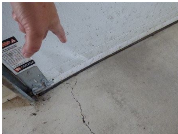
Bump in the garage door noted
