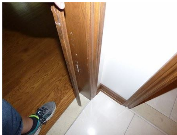
Frame is damaged. Repairs are needed.
